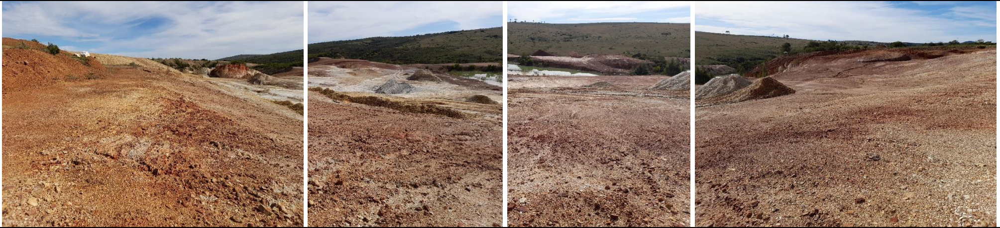
View of the Phase 1 mining area where the existing quarry (outside the mining footprint) can be seen at the back.
